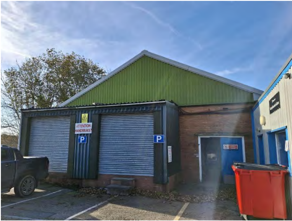
Photograph 15 – Building B: East aspect (front) of storage building. No bat roost potential found
