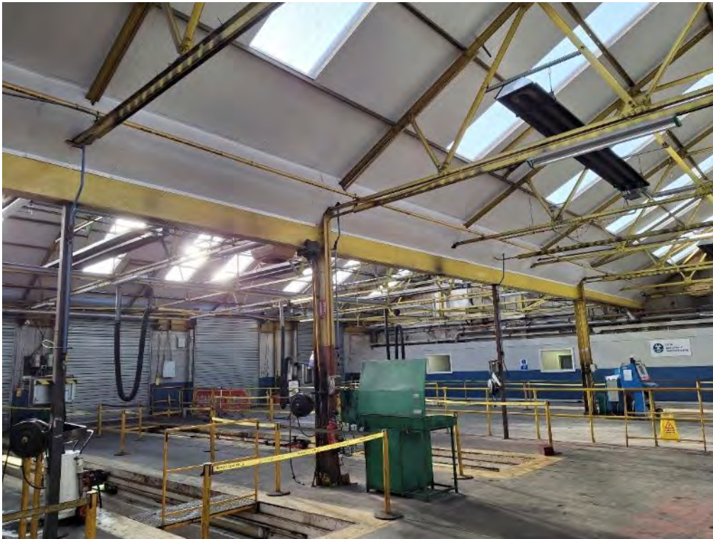
Photograph 13 – Building A: Interior of warehouse. Steel girders and concrete flooring with no potential bat roost features
